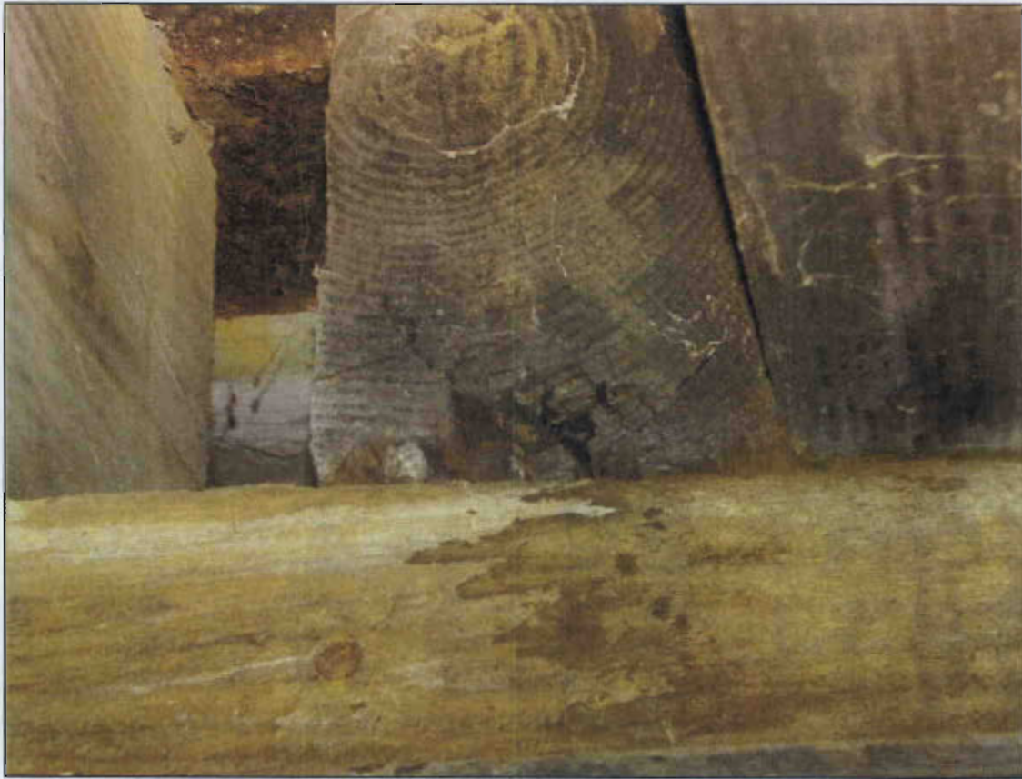
DECAY IN END OF JOIST 8 IN SPAN 1 OVER INTERIOR BENT
