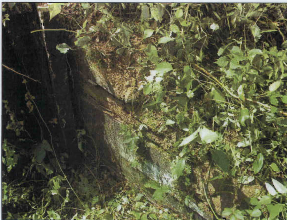
DECAY IN ENDS OF THE LEFT WINGWALL BOARDS AT END BENT 1
