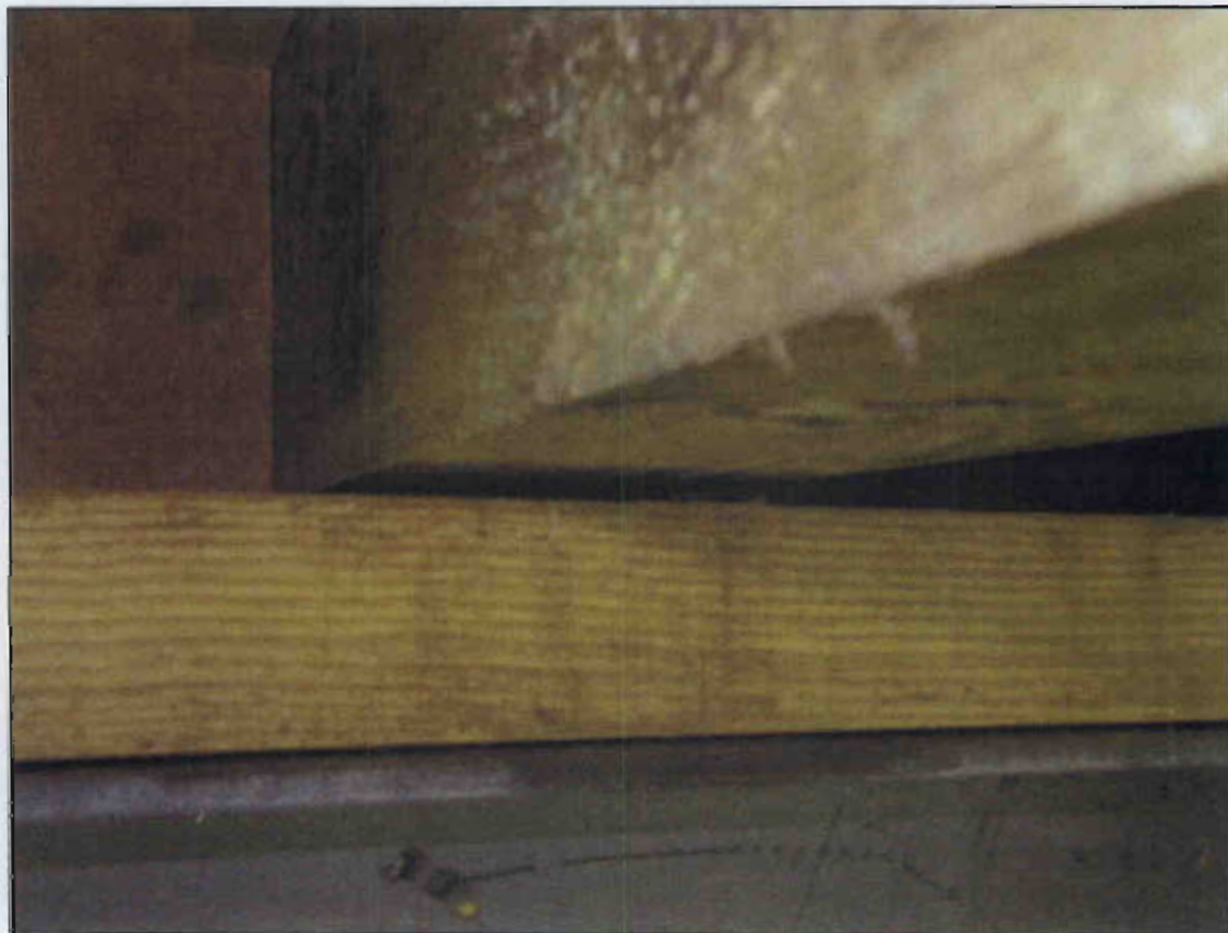
NO BEARING AT JOIST NO.18 OVER END BENT 2 CRUTCH (PRIORITY MAINTENANCE ISSUED)
