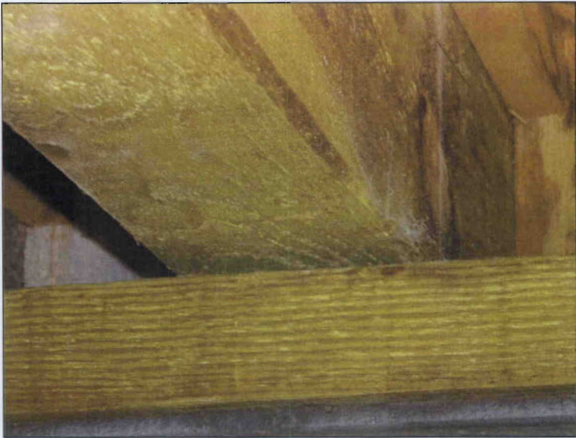
NO BEARING AT JOIST NO.17 OVER END BENT 2 CRUTCH (PRIORITY MAINTENANCE ISSUED)
