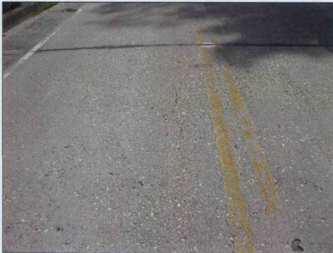
LONGITUDINAL CRACK IN THE LEFT LANE OF SPAN 1
