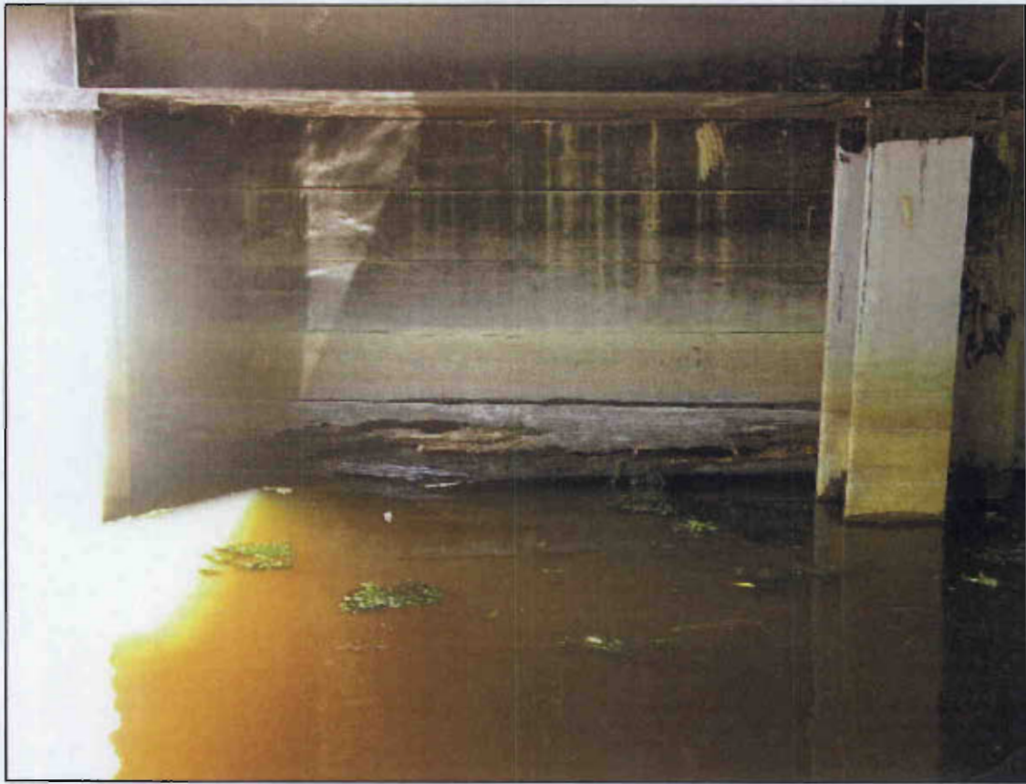
DECAY IN BULKHEAD BOARDS BETWEEN PILE 3 & 4 AT END BENT 1
