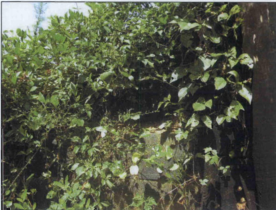
MISSING BOARDS FROM THE RIGHT WINGWALL AT END BENT 1
