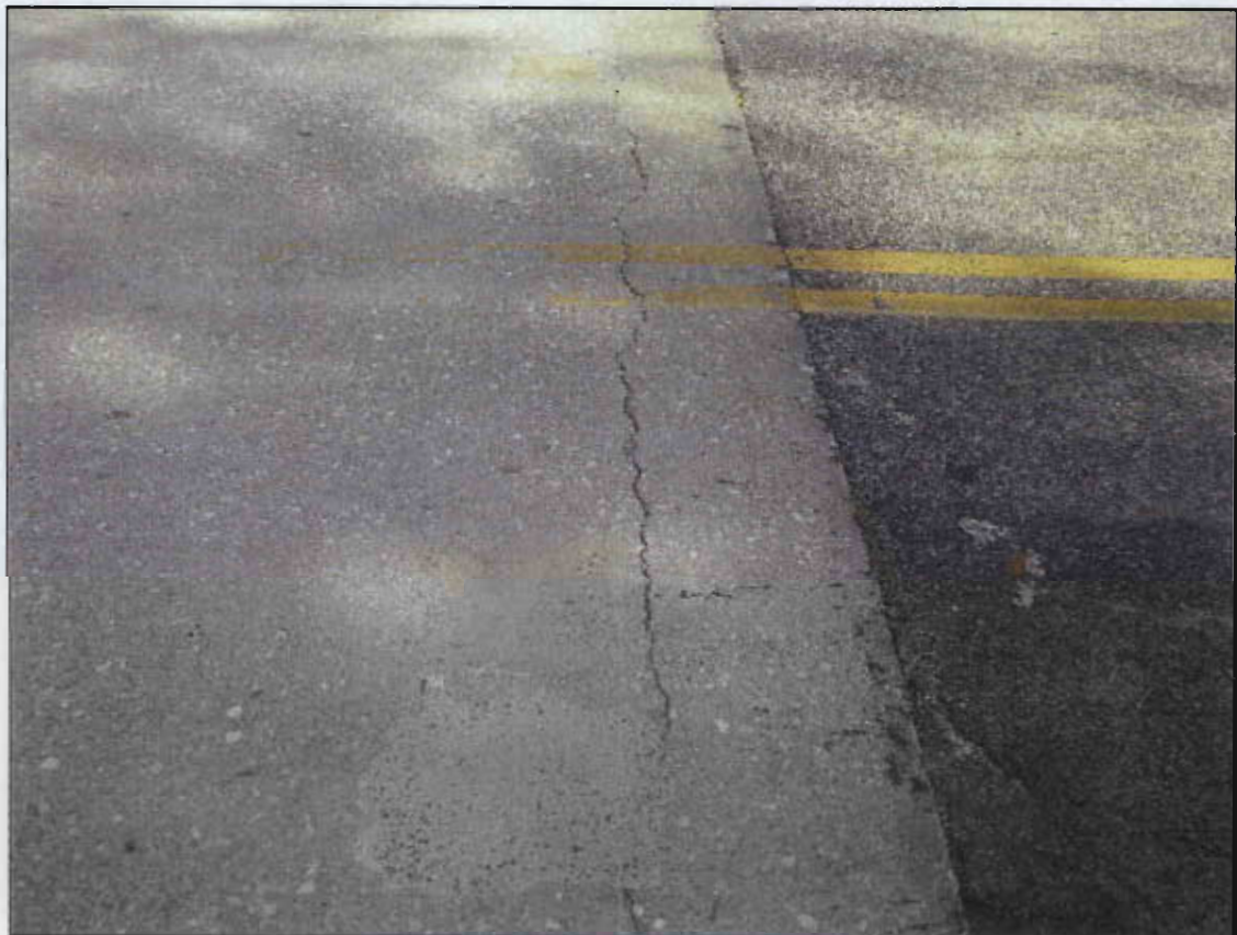
TRANSVERSE CRACK IN SPAN 2 AT END BENT 2
