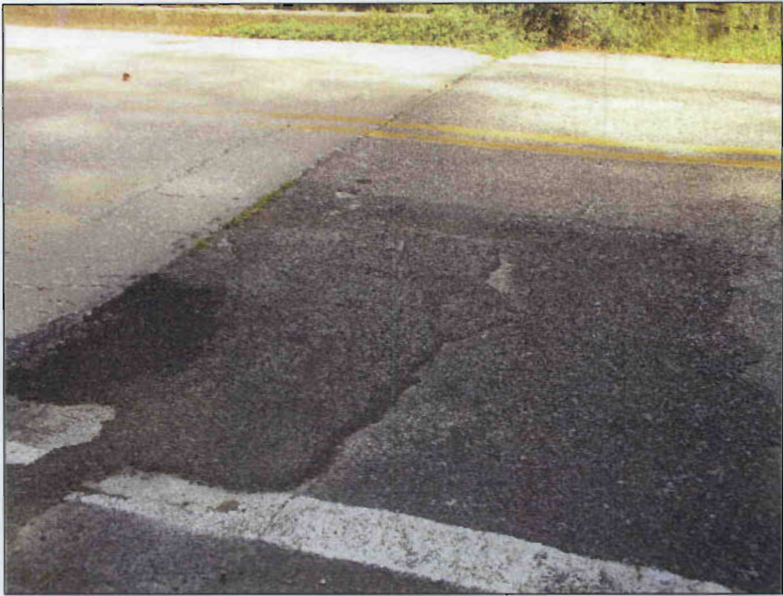
APPROACH 2 PATCHED AND SETTLED IN THE RIGHT LANE AT END BENT 2
