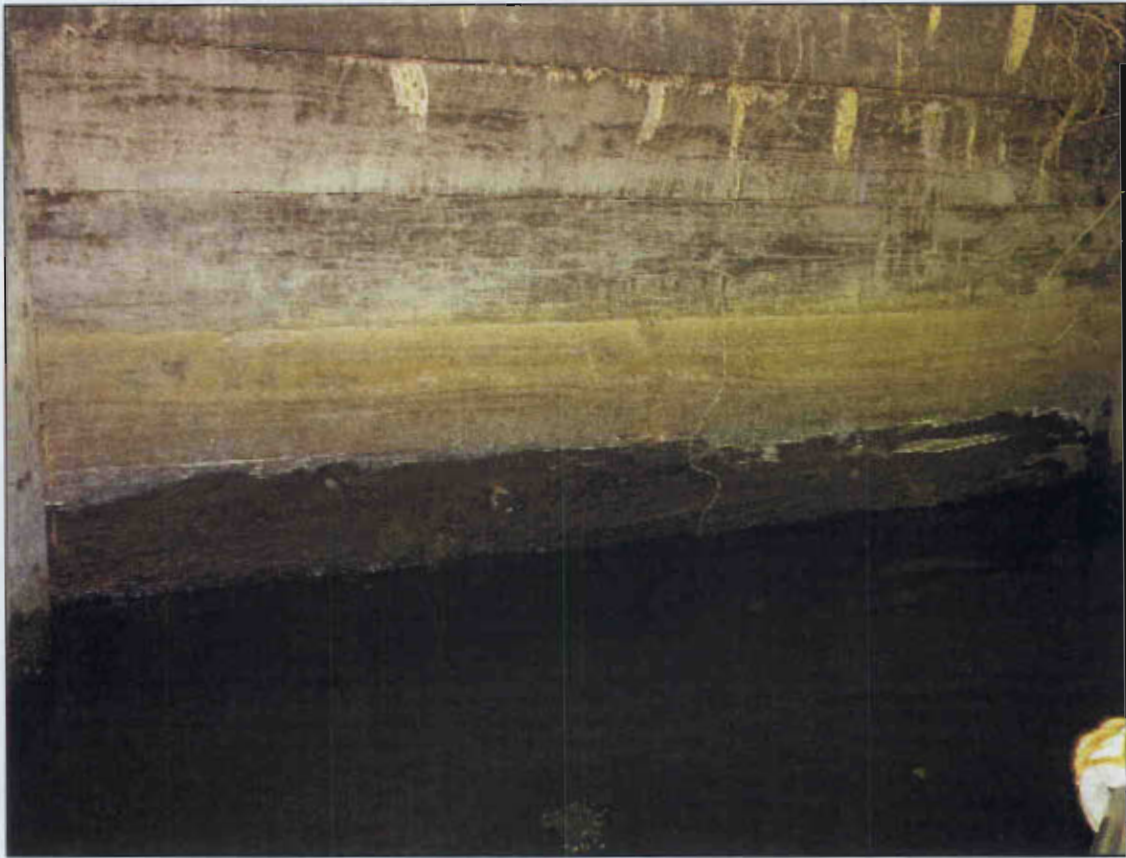
DECAY IN BULKHEAD BOARDS BETWEEN PILE 2 AND 3 AT END BENT 2
