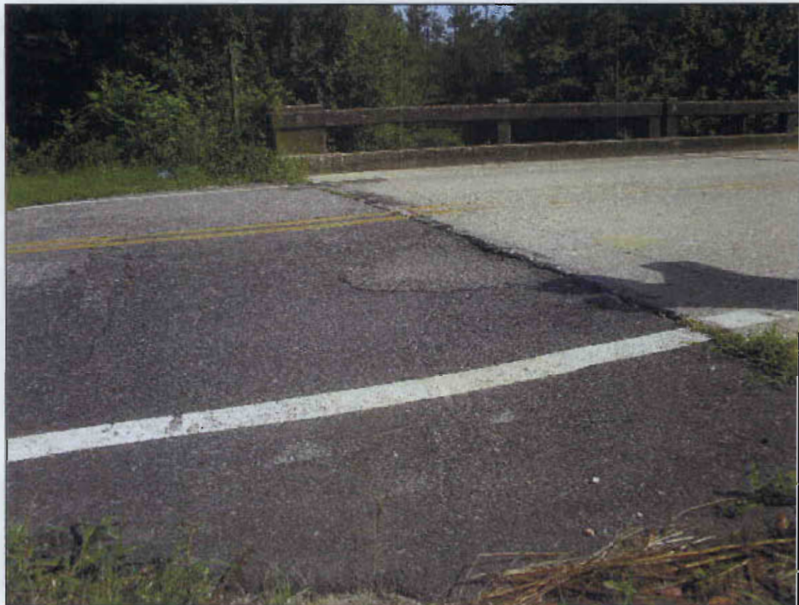
APPROACH 1 PATCHED AND SETTLED IN THE RIGHT LANE
