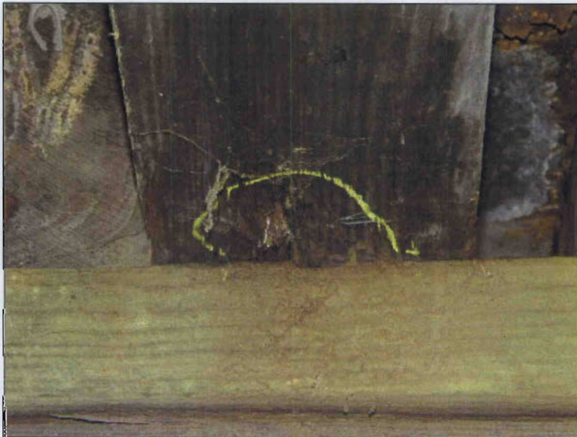
DECAY IN BOTTOM OF JOIST 5 IN SPAN 1 OVER INTERIOR BENT
