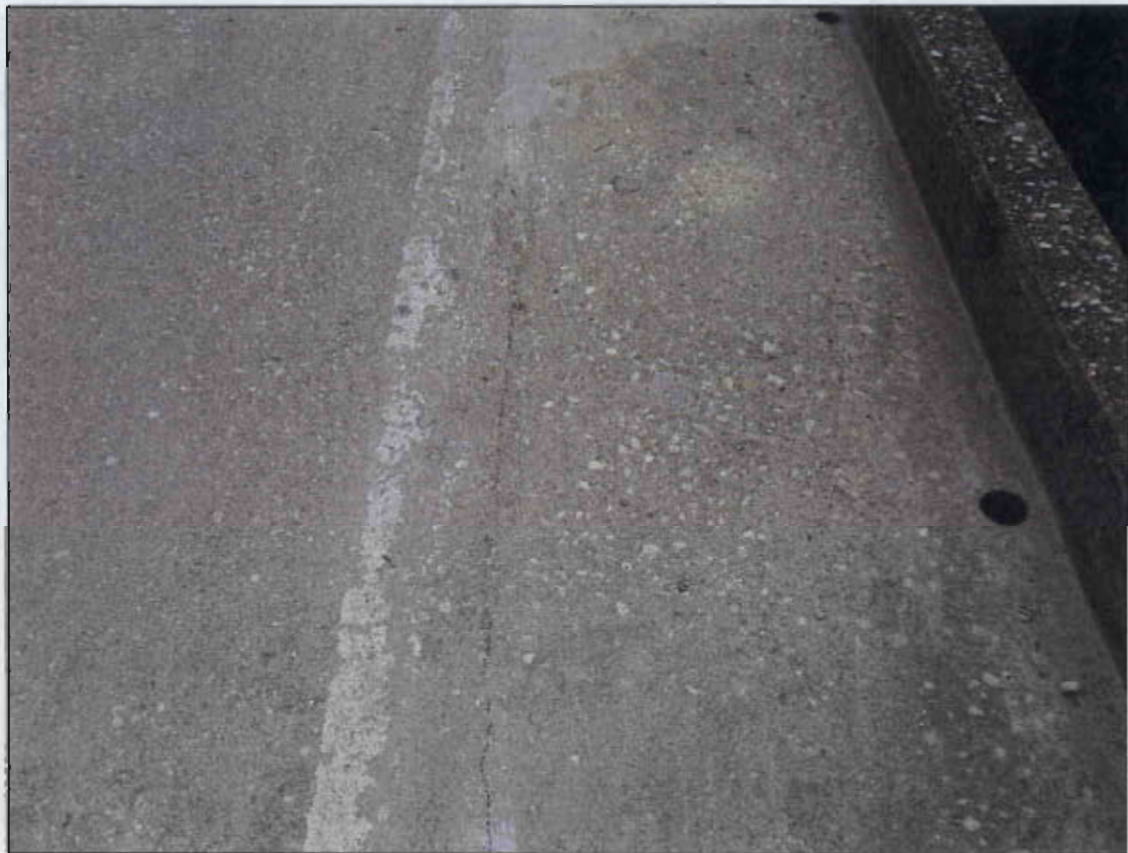
LONGITUDINAL CRACK IN THE RIGHT SIDE SHOULDER OF SPAN 2
