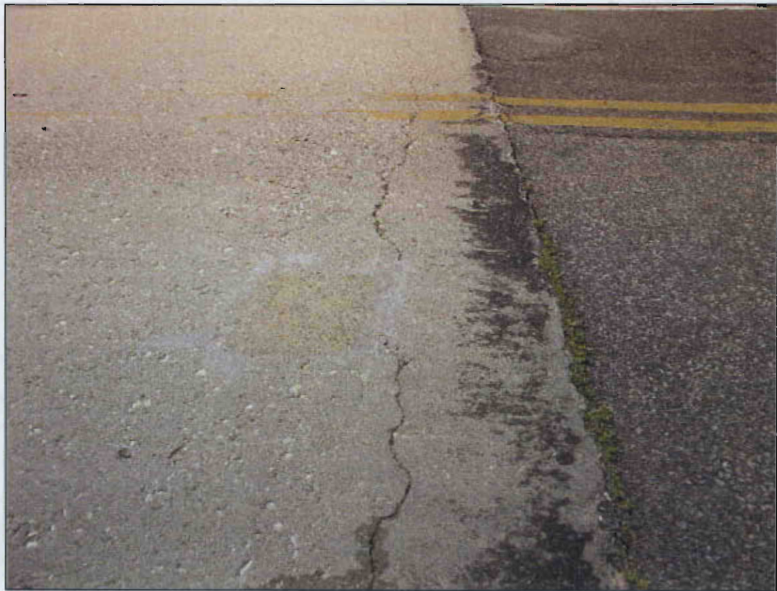
TRANSVERSE CRACK IN TOP OF DECK AT END BENT 1
