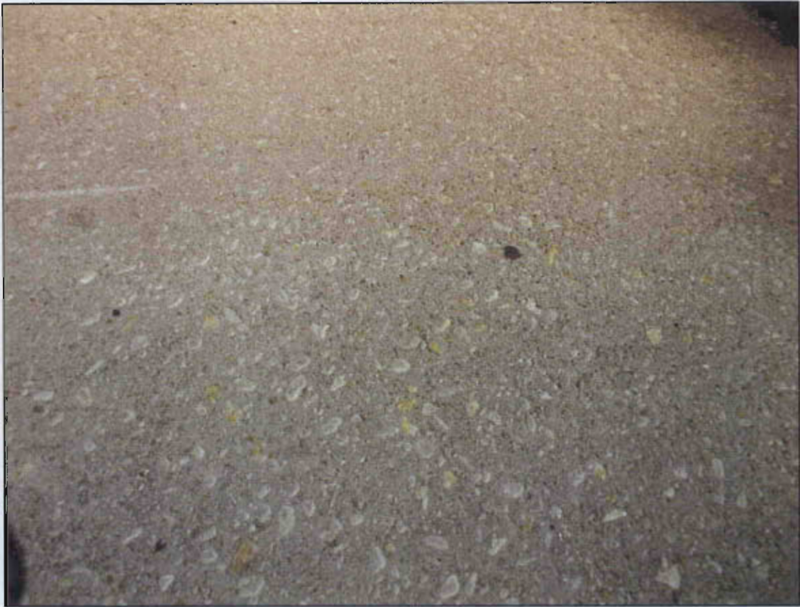
TOP OF DECK SCALED WITH COARSE AGGREGATE EXPOSED
