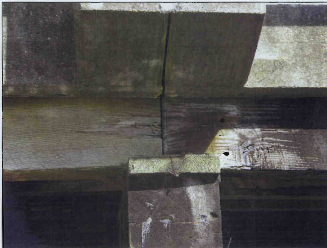
MISSING SPLICE BLOCK AT THE RIGHT SIDE OF INTERIOR BENT
